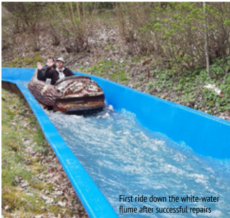
Work in progress: MC-DUR TopSpeed in combination with the polyester nonwoven MC-Floor Tex
