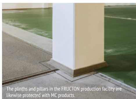
The Polish food producer FRUCTON opted for the exceptionally resilient MC-DUR PowerCoat 280 industrial floor in green, capable of withstanding temperatures of up to 120 °C.
